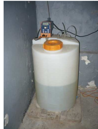
Figure 3-18 Disinfection with sodium hypochlorite in Govedare PS
