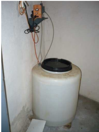
Figure 3-16 Disinfection with sodium hypochlorite in Ognyanovo PS
