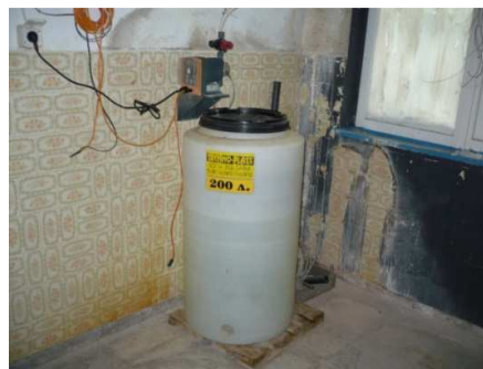
Figure 3-13 Disinfection with sodium hypochlorite in Zvanichevo PS
