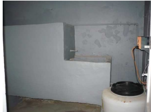
Figure 3-15 Disinfection with sodium hypochlorite in the chlorination facility next to Sinitevo PS
