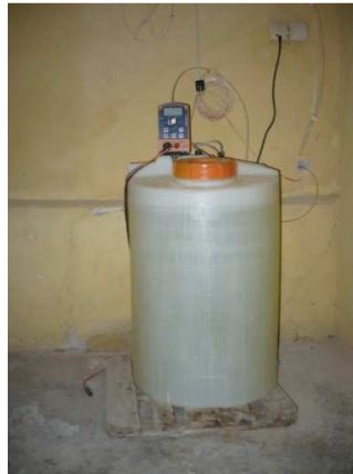
Figure 3-17 Disinfection with sodium hypochlorite in Hadzhievo PS
