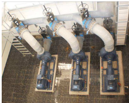
Figure 3-39 WWPS Industrial water
