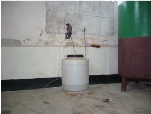
Figure 3-14 Disinfection with sodium hypochlorite in Lyahovets-Bratanitsa PS
