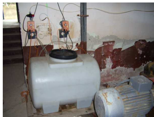
Figure 3-21 Disinfection with sodium hypochlorite Dinkata PS
